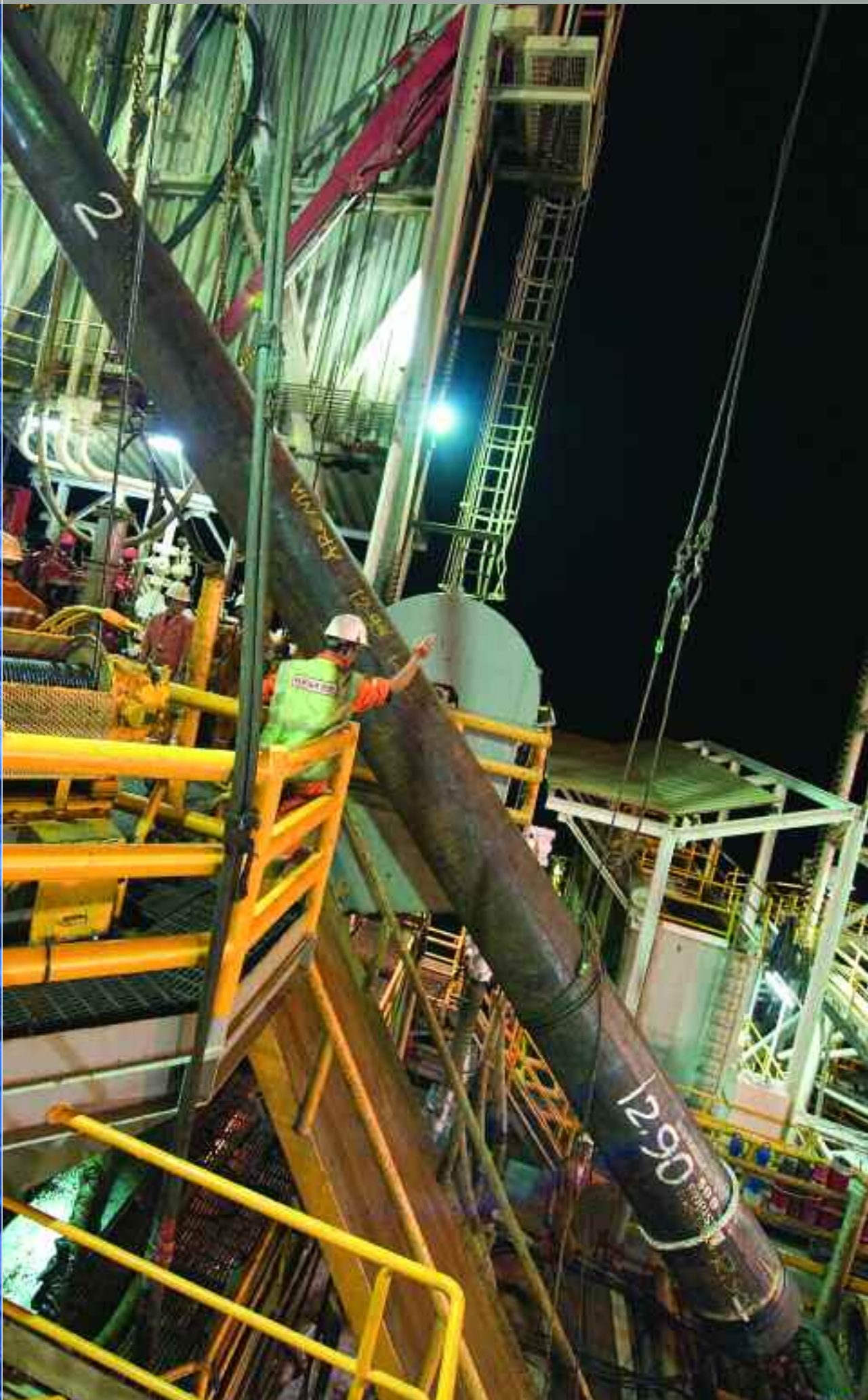
A length of 30 inch conductor pipe is being winched into the drilling rig derrick ready to be installed in a Kambuna development well. Conductor pipe is the outer casing used in drilling a well. The casings provide a means of circulating drilling mud to surface to remove rock cuttings as the well is drilled.
